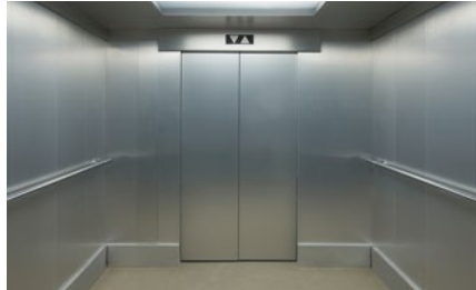
Lifts &amp; escalators
